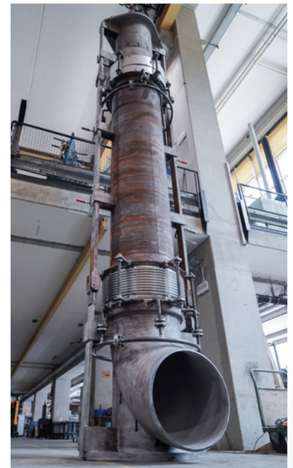
8 metres long and 3.2 tons in weight – a lateral expansion joint in maintenance
