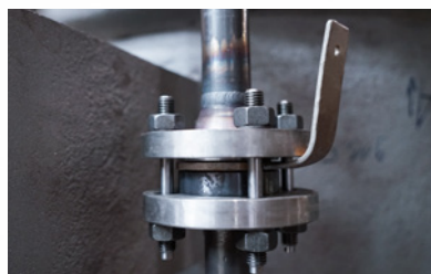
Adjustment orifice plate for regulation of the amount of steam for the injection
