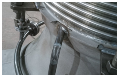
Ring line for the injection. This prevents the bellows becoming carbonised and reduces the bellows temperature
